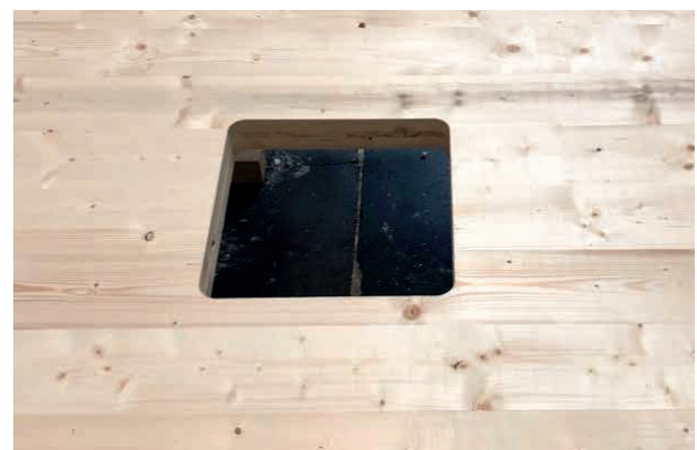
Cut-out, residual radii not removed
