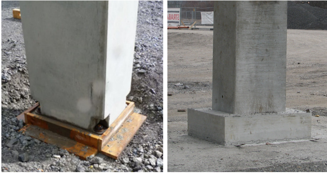
Figure 2. Formwork in readiness for grouting (left), finalized connection after grouting has hardened (right).
