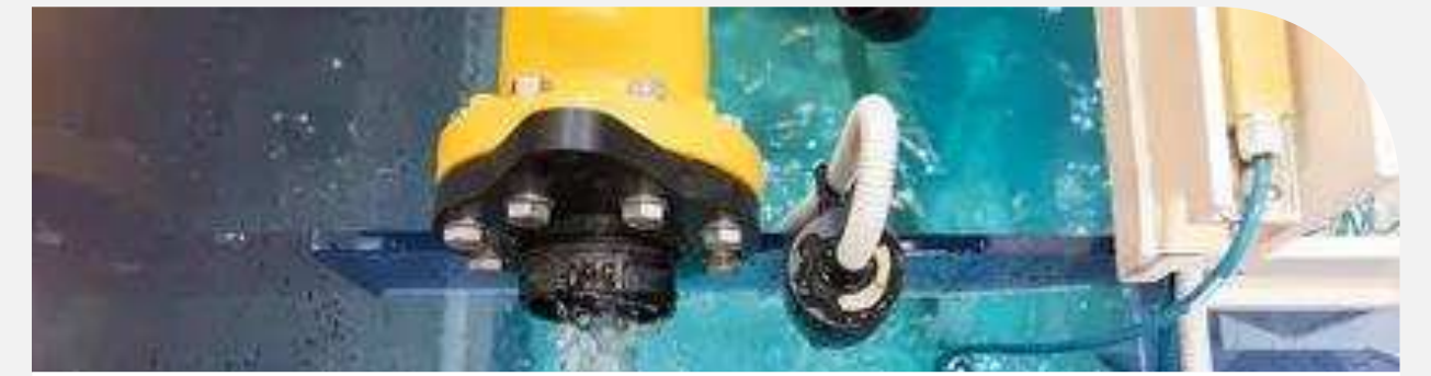
Management of water & sewage plants
